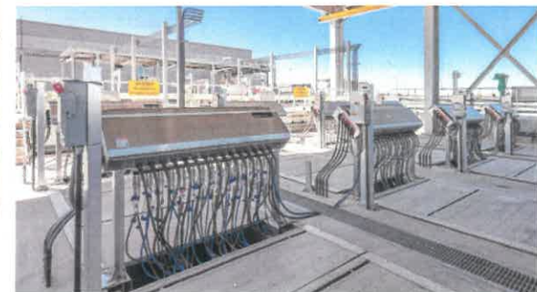
New UV Reactor in Channel 4
